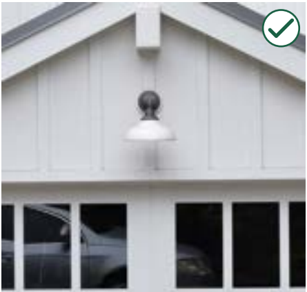
Locate and shield fixtures to avoid glare.
