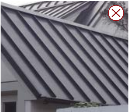
Standing seam metal (inappropriate)
