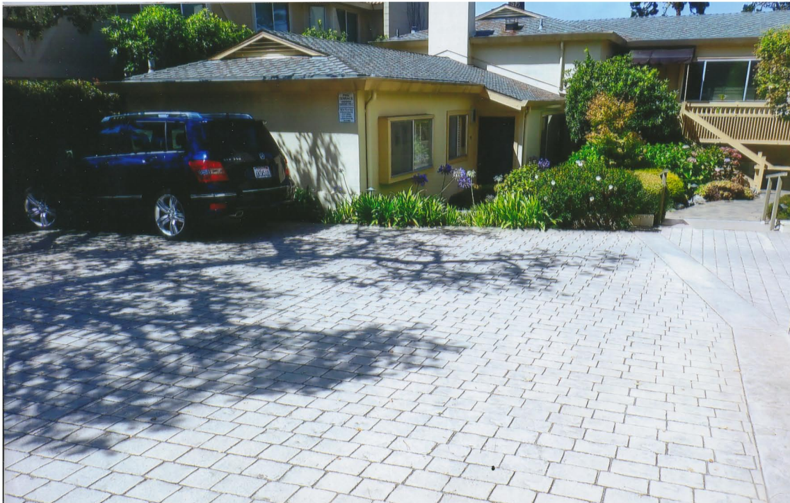
Photo #3. Looking SW from Mission St., Note c. 2007 paving changes, & c. 1980 Comp Roofing on Bldg D. Kent Seavey, Sept., 2025.
