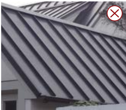
Standing seam metal (inappropriate)
