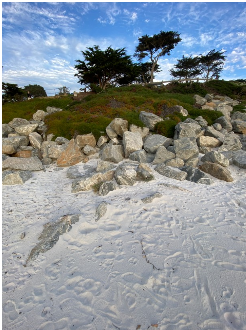
Photograph 48: Revetment R3 Showing Area of Rip-rap on December 22, 2022 Where the Public Could Benefit from Quarystone Re-stacking
