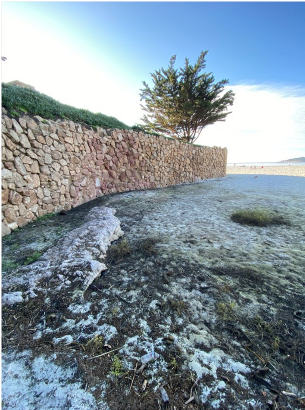
Photograph 22: Southern End of Seawall S3 on December 22, 2022
