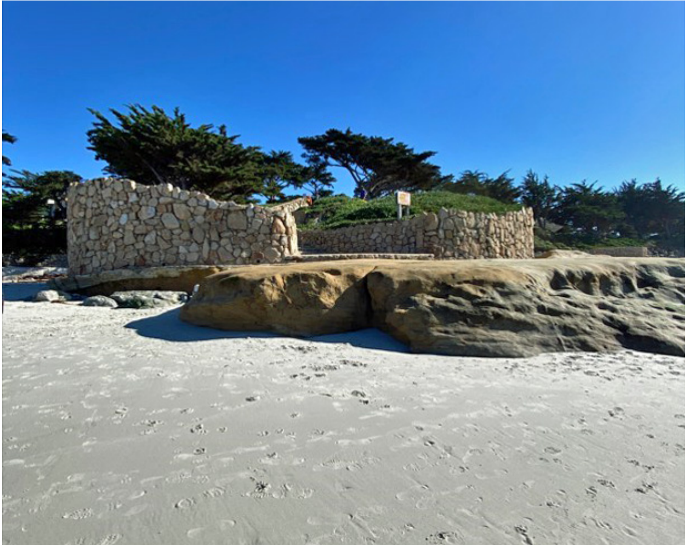
Photograph 28: Showing Public Access Stairway ST3 with Seawall S3 on Both Sides On January 30, 2023
