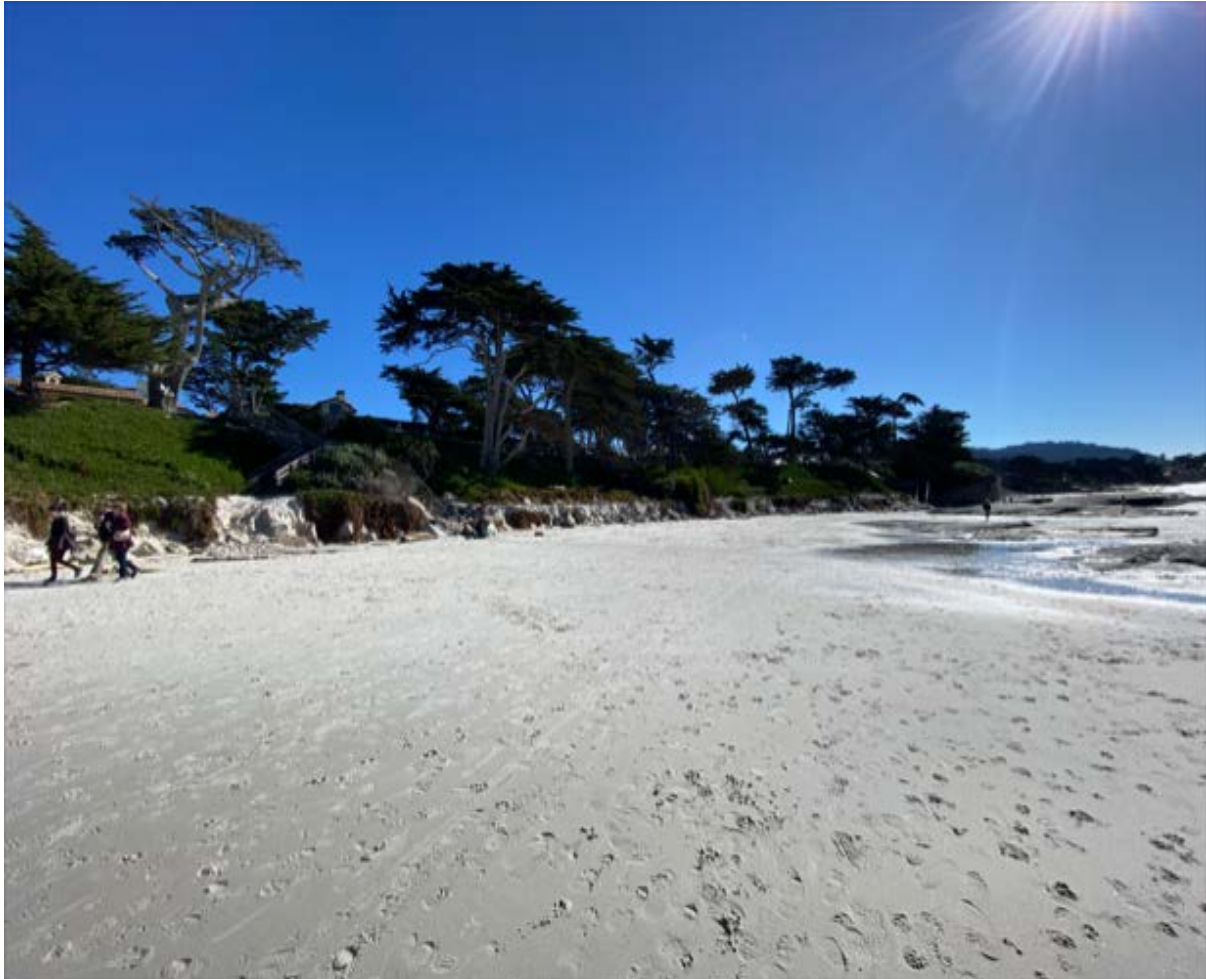
Photograph 78: Central Portion of Revetment R5 on January 30, 2023
