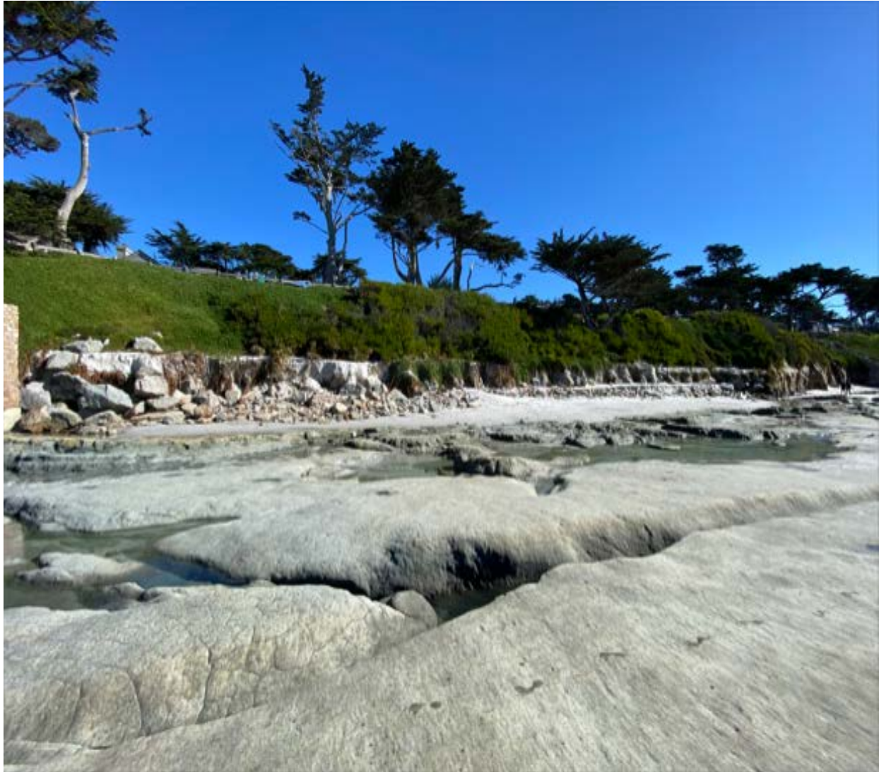
Photograph 62: Northern 1/3 of Revetment R4 Showing Very Undersized Scattered Rock on January 30, 2023
