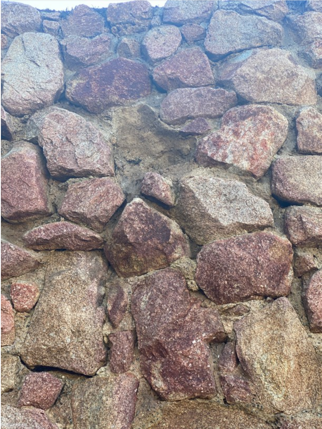
Photograph 26: Seawall S3 Showing Missing Rock on December 22, 2022
