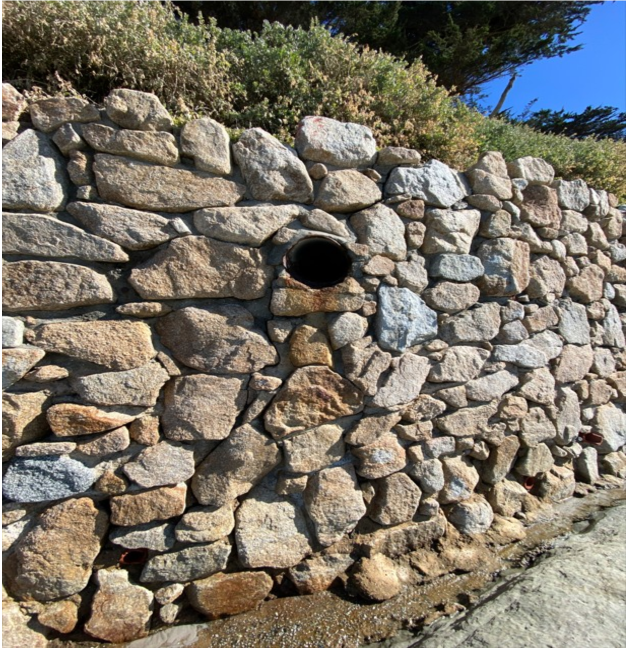
Photograph 72: Storm Drain in Seawall S7 on January 30, 2023
