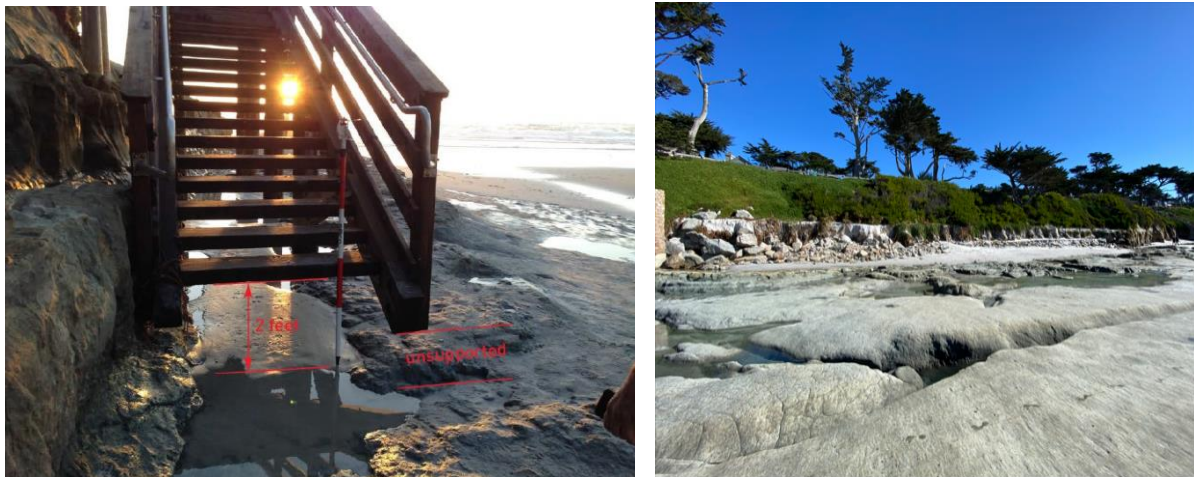
Figure 1. Left, undermined 12th Avenue stairway following the El Niño Winter of 2015–16 (January 24, 2016). Source: Easton Geology (2016) Right, the beach scoured down to bedrock near 10th and 11th avenues following strong winter storms of 2022–23 (January 30, 2023). Source: HKA (2023).
