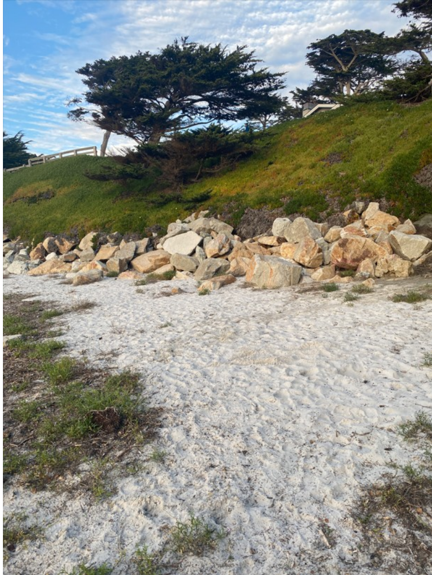
Photograph 47: Revetment R3 Showing Scattered Rip-rap Boulders on December 22, 2022
