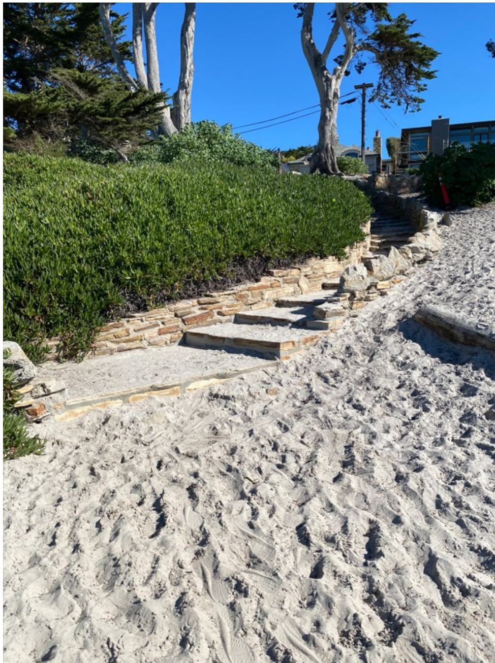
Photograph 87: Toe Conditions at Seaward End of Stairway ST9 on January 30, 2023
