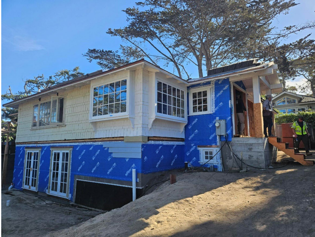
Figure 2: View of new windows on the front elevation and missing horizontal siding.
