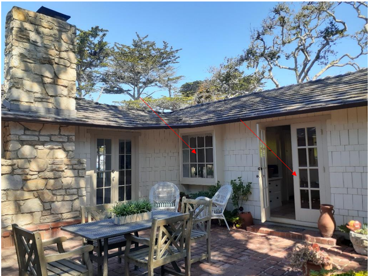
Figure 2: Arrows indicate window and French doors that will be removed on the north side of the courtyard.
