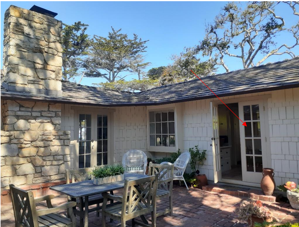
Figure 6: View NW of patio and French doors added in 1950, indicated with red arrow
