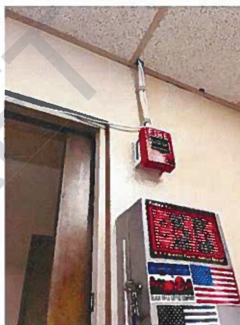
Figure 40 - Existing Manual Pull Station
