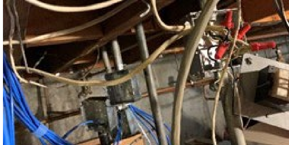
Electrical box missing cover
