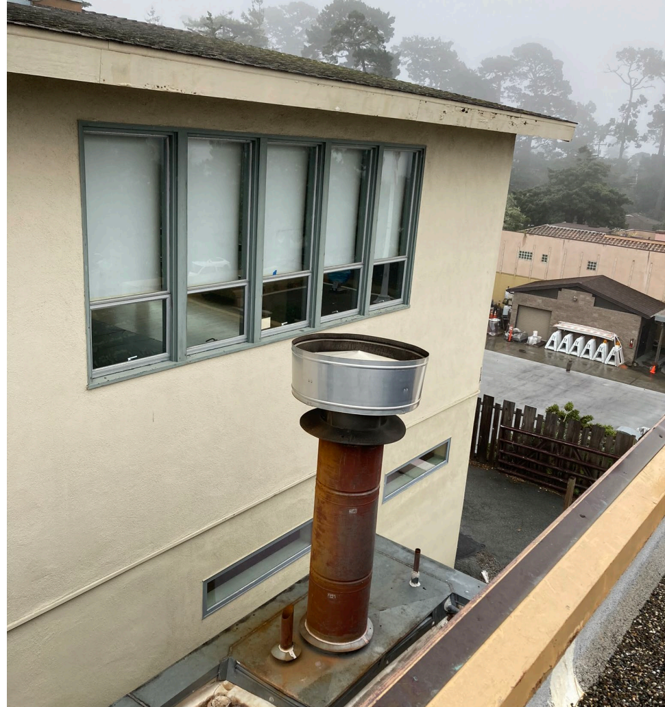
Non-Compliant boiler exhaust
