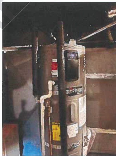
Figure 41 – Existing Hot Water Heater (No Expansion Tank)
