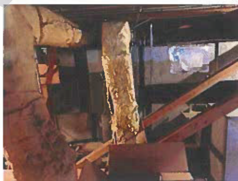
Figure 48 – Existing Duct Insulation
