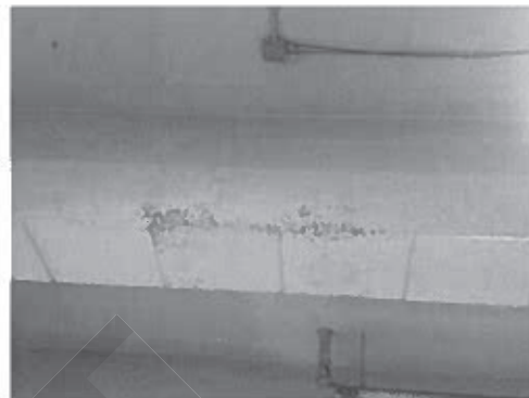
Figure 13 – Rock Pockets in Existing Parking Structure
