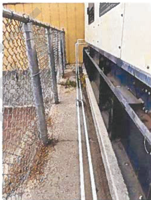
Figure 37 - Clearance in front of existing generator
