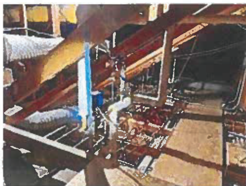
Figure 32 – Electrical splices not in electrical box.
