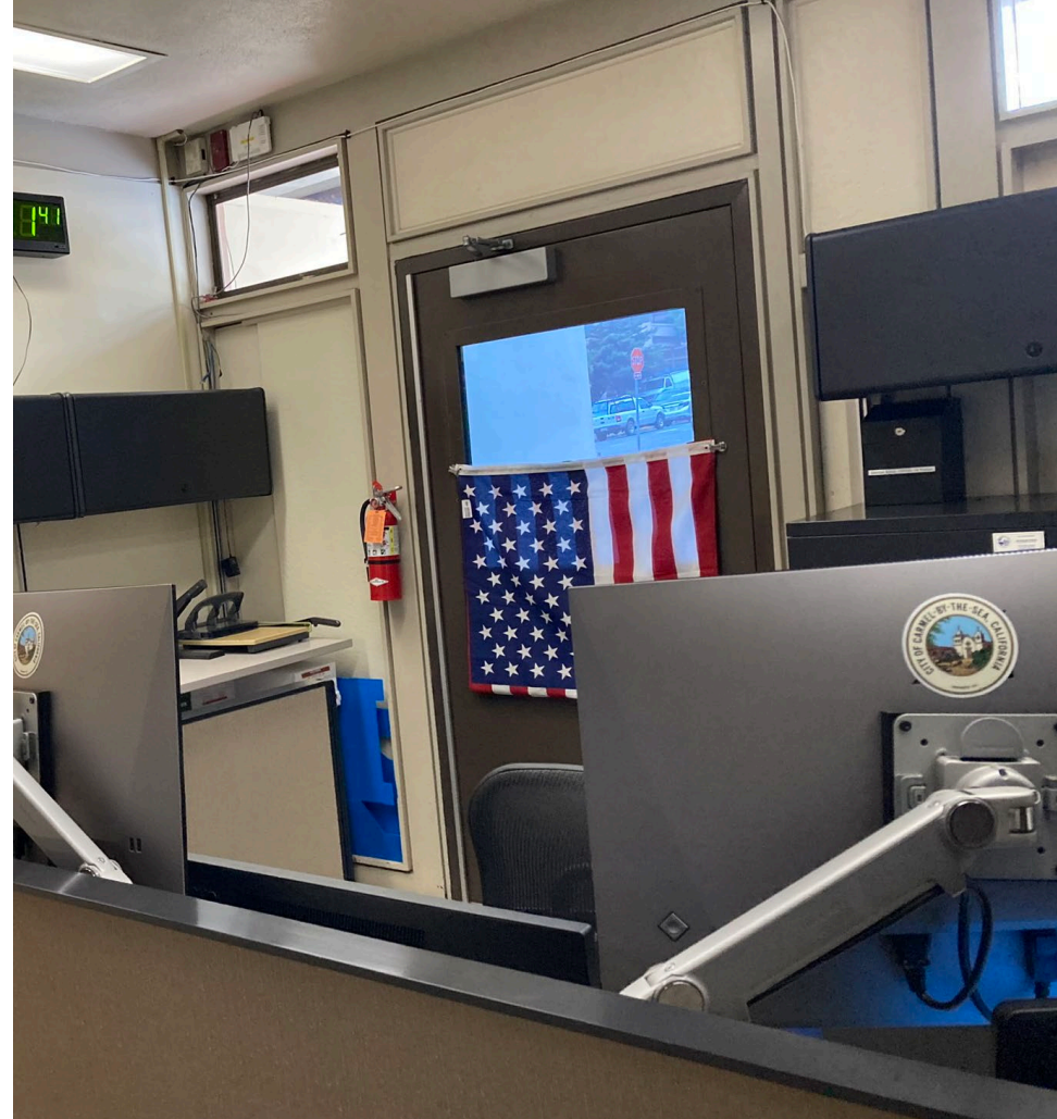
Non secure door at dispatch leading to unsecured parking area
