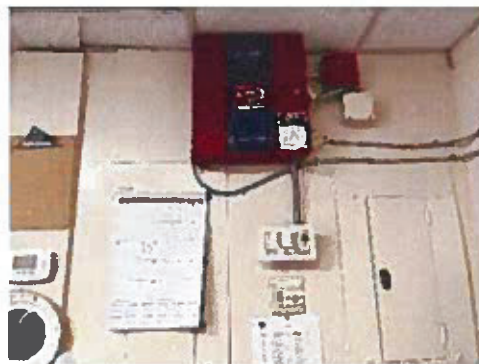
Figure 39 - Existing Fire Alarm Control Panel
