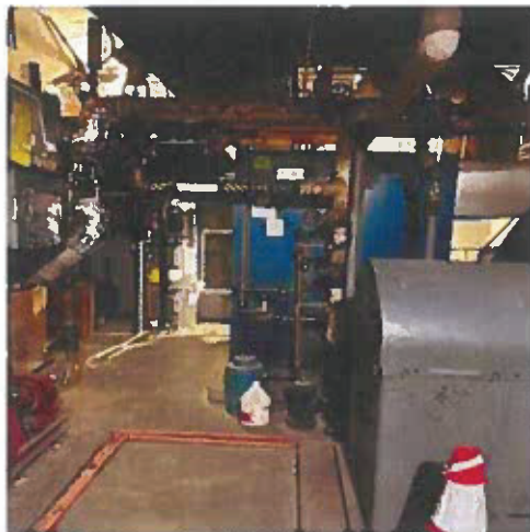
Figure 17 - Existing Hot Water Boiler (Mechanical Room)
