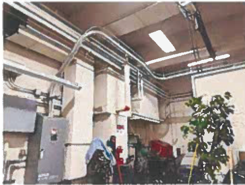
Figure 23 – Existing Hot Water Pipes Over Transfer Switch
