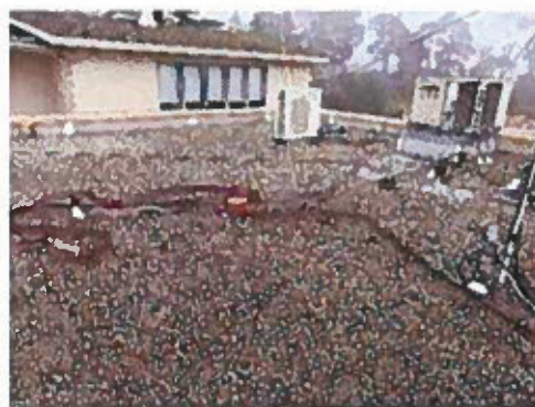
Figure 33 – Existing disconnected lightning protection
