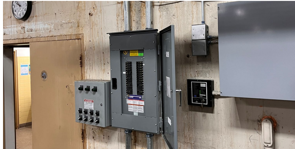
Water intrusion at electrical equipment
