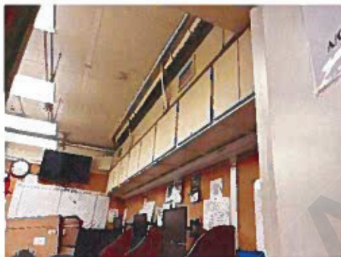
Figure 28 – Existing Shooting Range Supply Ventilation
