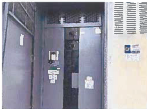
Figure 38 - Existing power distribution switchboard
