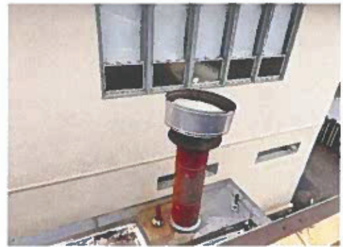
Figure 22 – Existing Hot Water Boiler Flue
