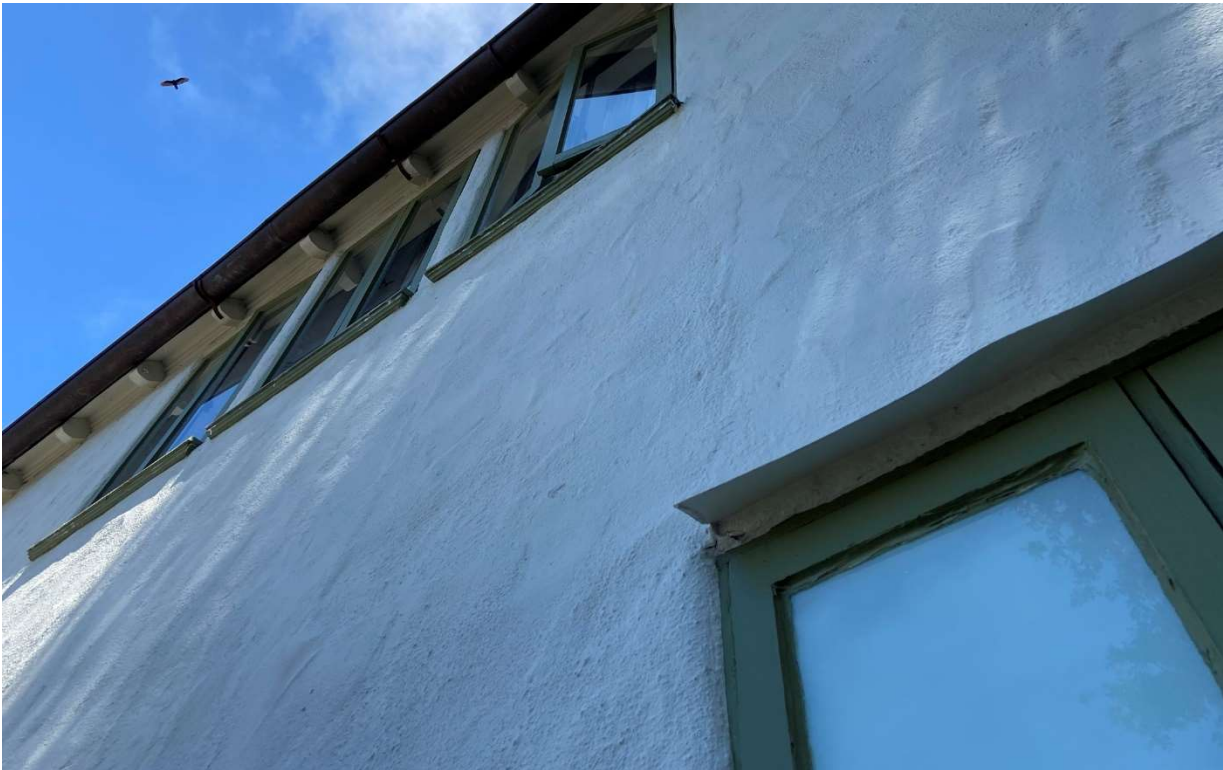
Photo #12, bent/damaged flashing at second level opening
