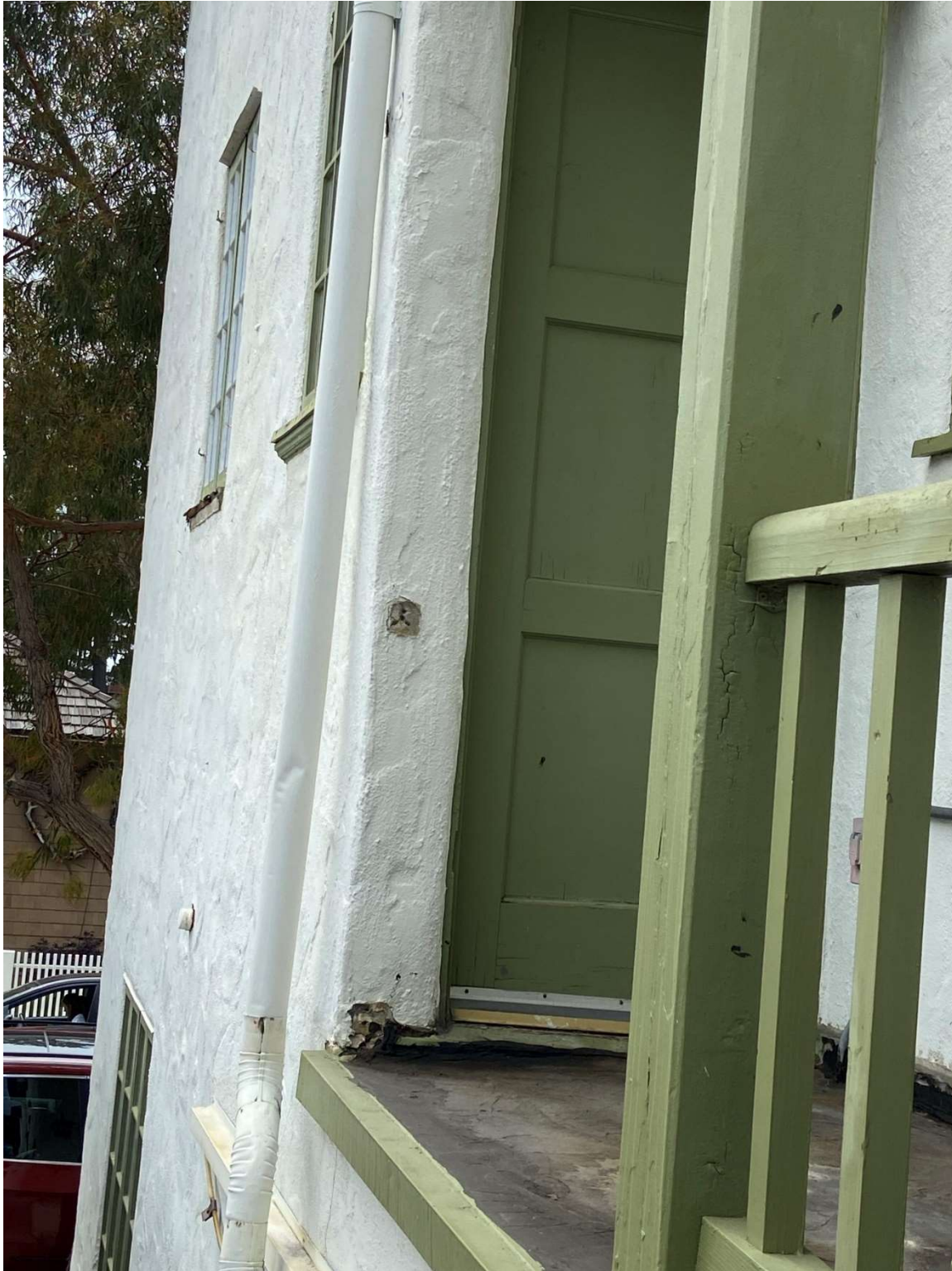
Photo 14, Water damage at upper-level balcony
