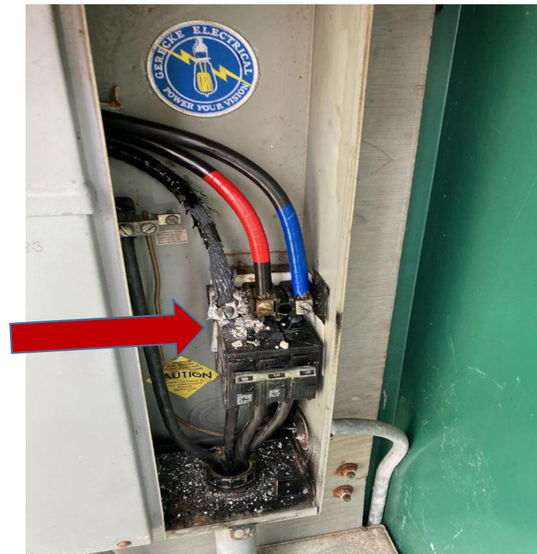
North Lot Electrical Panel
