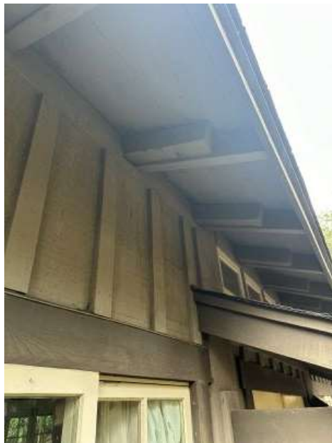
Figure 6 Structural rafters too short
