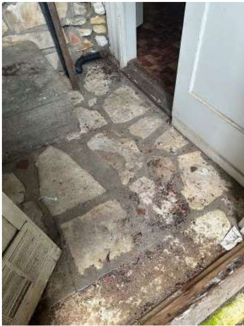
Figure 24 Masonry floor touching wood elements
