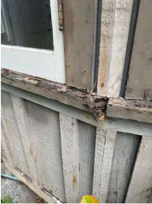
Figure 21 Termite damage at window sill
