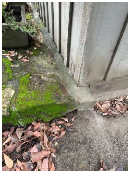
Figure 2 Patio contacting wood siding
