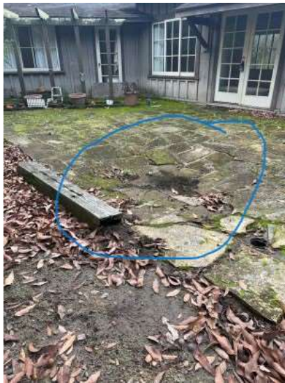
Figure 1 Area of patio subsidence
