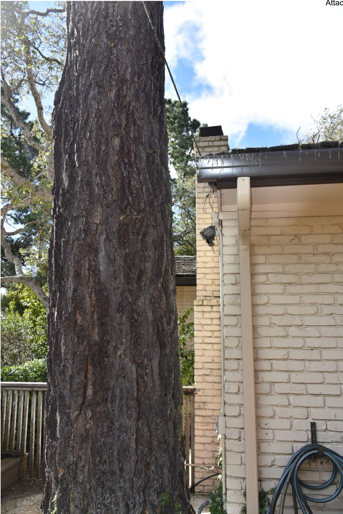
The proximity of the tree to the house
