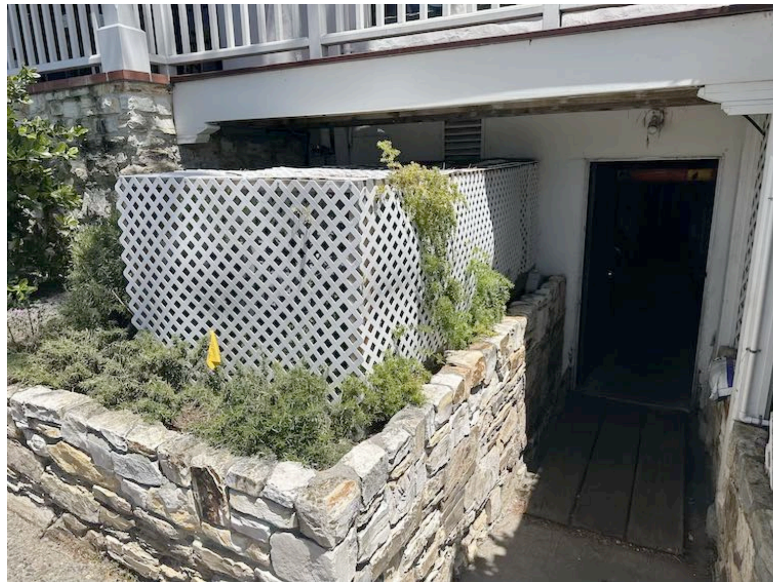
Existing Gas Meters and Screening and Mechanical Room Walkway at Monte Verde Street
