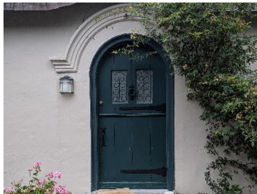
Front door to be restored.
