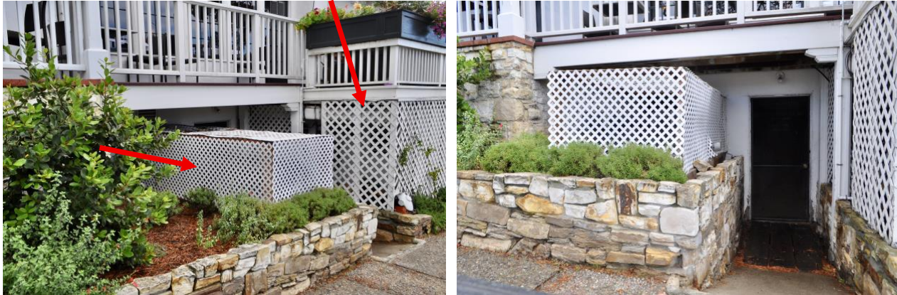
Figures 3 and 4. Left image looks south down the Monte Verde St. sidewalk at the existing locations of the fire sprinkler infrastructure. Left arrow shows a plastic lattice screen added after 2002 in an effort to match the wood lattice screen installed during the 2002 Thodos remodeling campaign (right arrow). Right image views the lower utility room entrance and the two areas impacted.
