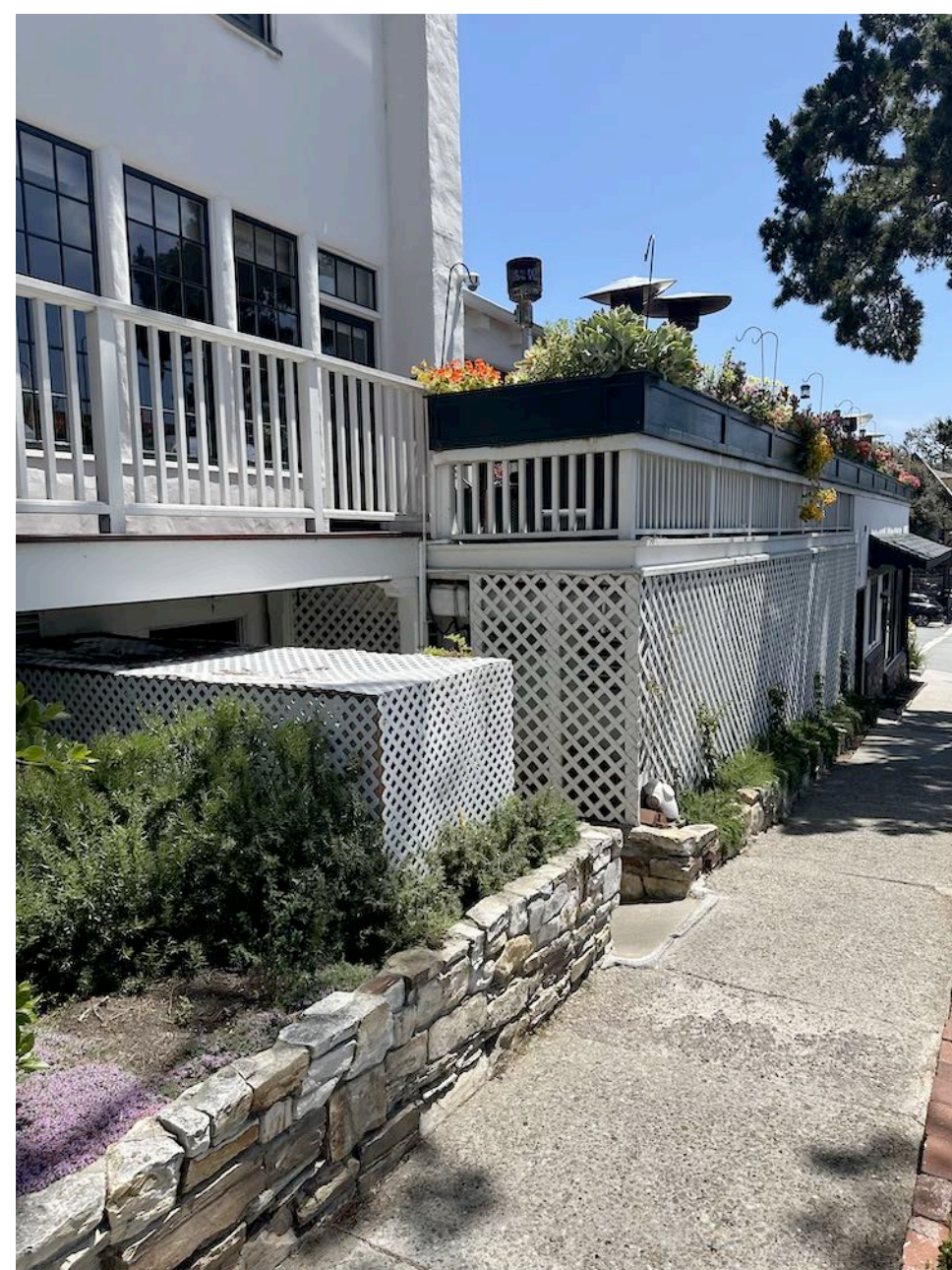
Existing Gas Meters and Screening at Monte Verde Street
