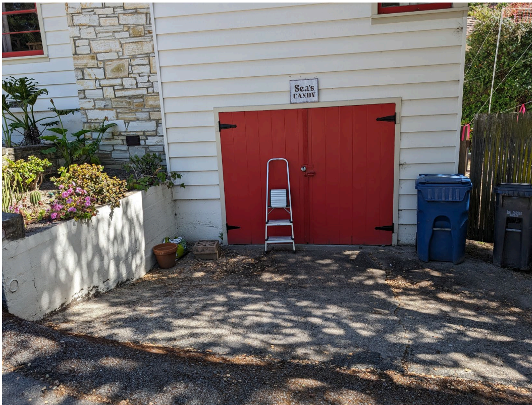
Garage door to be modified and opening to be enlarged. Original garage door pictured.
