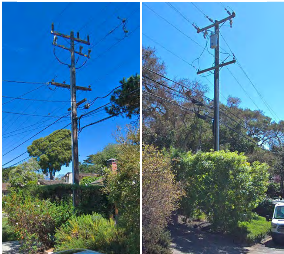
Infeasible Utility Poles in A-1 Zone Behind Golden Bough Playhouse, Casanova Street
