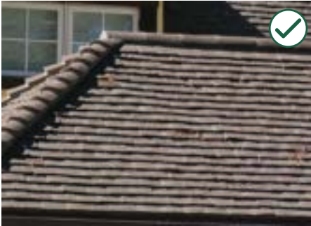
Clay roof tiles
