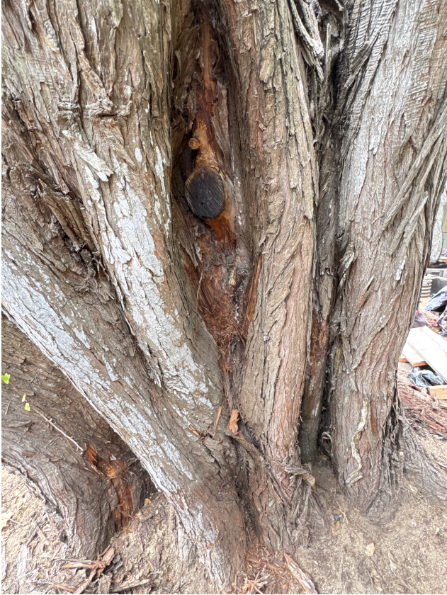
Advanced decay and vertical reaction wood forming - The presence of well-developed vertical reaction wood shows the tree has been long-standing and is under chronic mechanical stress.
