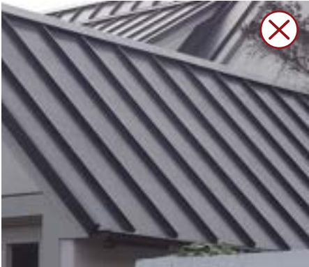
Standing seam metal (inappropriate)
