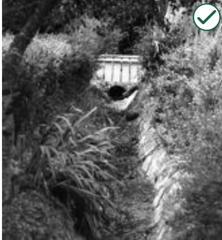
Maintain the existing character of street gutters in each neighborhood.
