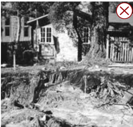
Excavation work shall be planned to avoid significant impacts to root systems. As shown here, cutting into major roots systems without City approval will weaken or even kill a tree and is unlawful.
