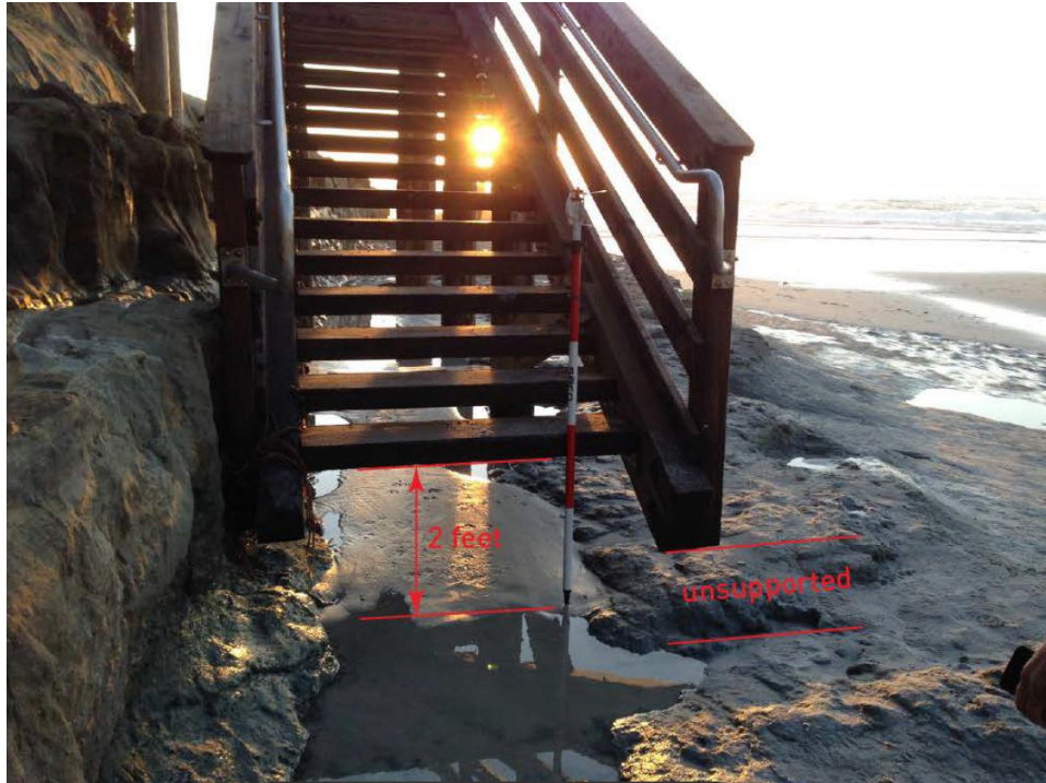
Figure 41. Gap at Bottom of 12th Avenue Stairs (Easton Geology 2016)
