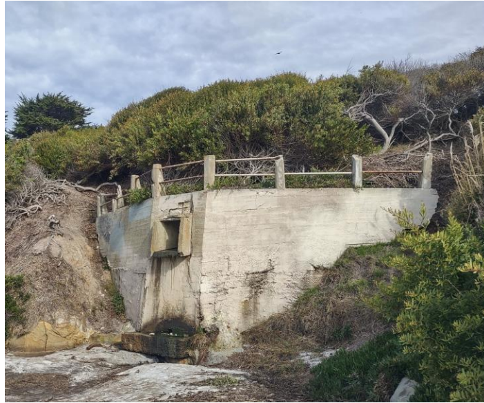
Figure 31. 4th Avenue Seawall and Outfall
