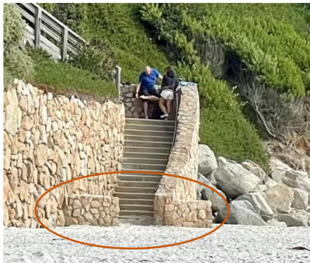
Figure 17. Wave Deflectors at the Base of a Beach Access Stairway
