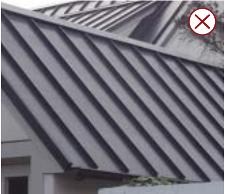
Standing seam metal (inappropriate)
